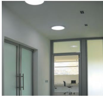
Daylighting system Almecco offices in Milan
